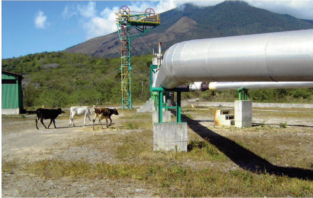
Figure 8.1 Typical pipeline at Miravalles geothermal power plant, Costa Rica (photo by R. DiPippo).
